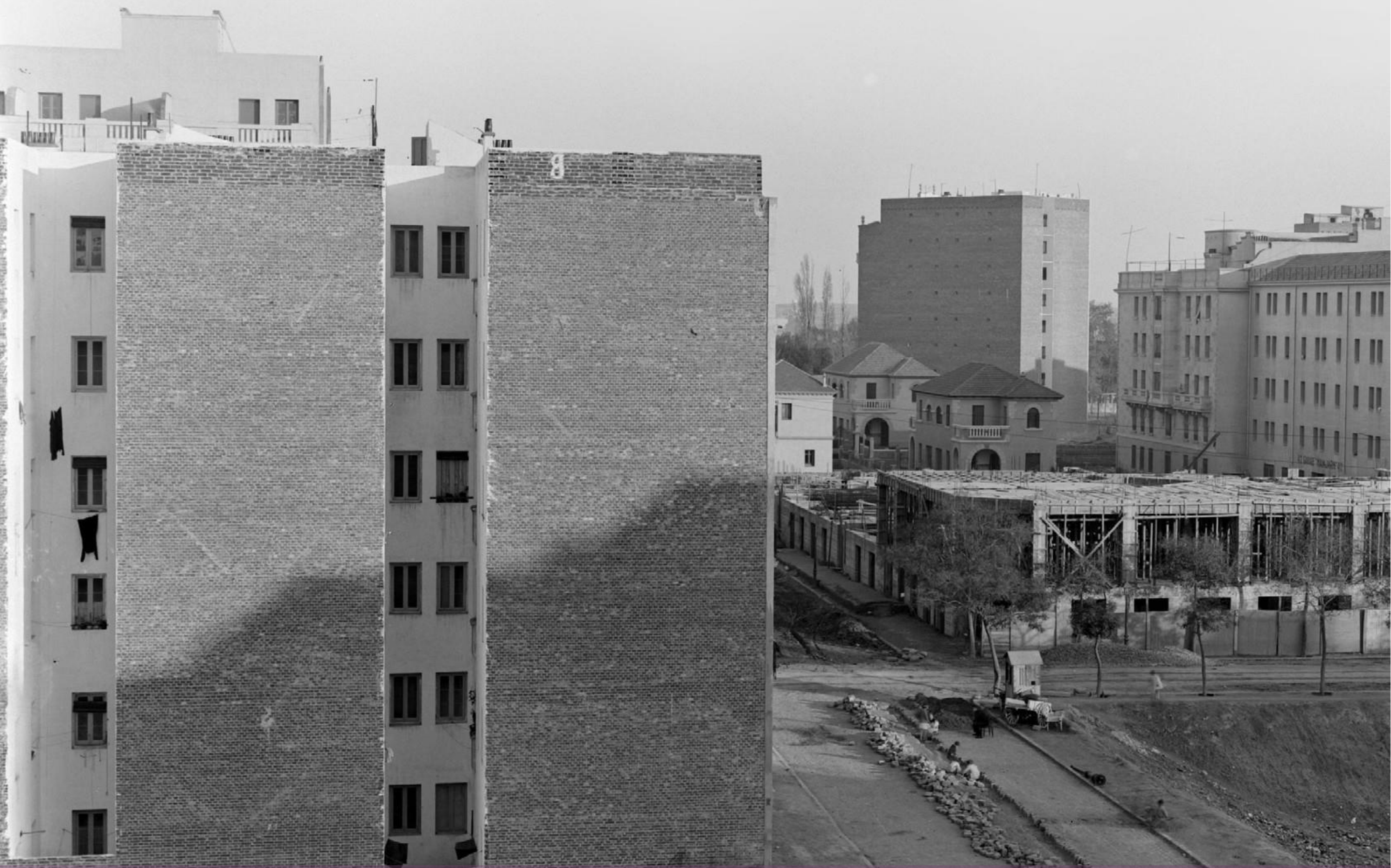
Housing under construction, Royal Co-operative Institution for State, Provincial and Municipal Officials, c/ Padilla, 76-82, Madrid. Foto: E. Ferrés y L. Lladó, H. 1920-30, Simurg, Fondo digital del CSIC.
